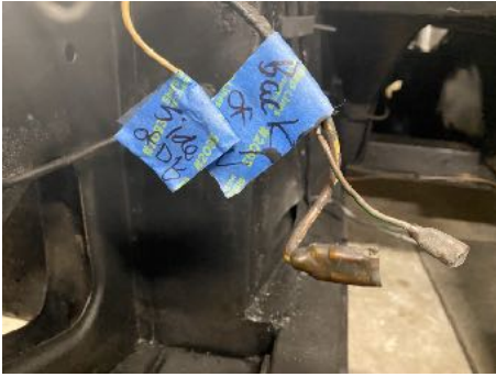
Tape flags work perfect for wires as well. Kyle Smith
