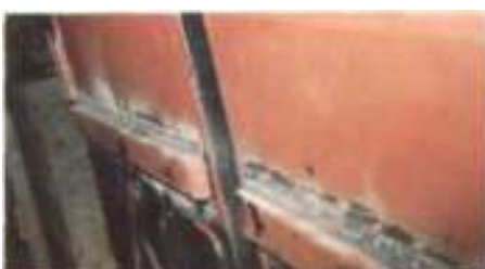
Underside after floor repair completed and prior to fitting of new jacking-point.
