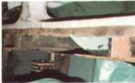
All the unground metal removed.
