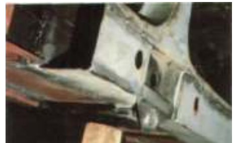
Showing relationship Between new jacking-point and already completed work on floor and sills.
