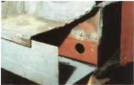
Front of offside side-beam showing how new parts have been fitted and prior to final finishing. The section with the circular ventilation hole is part of the new half-inner-sill panel and the L-section the new 14-gauge panel to replace the outer and lower parts of the beam.
