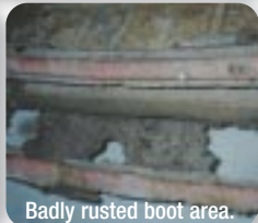
Badly rusted boot area.
